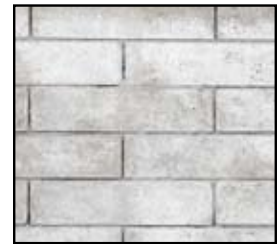
Refractory Brick Liner
